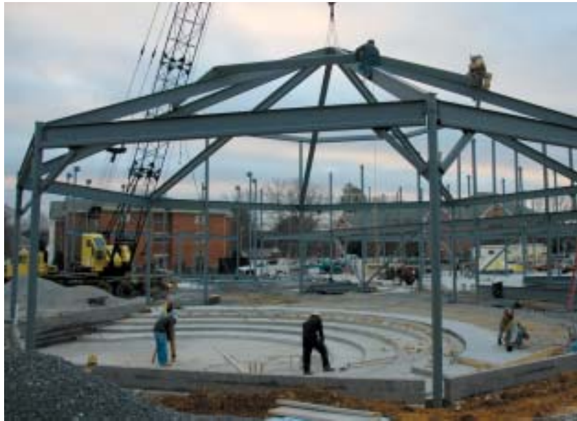
Welders, riveters and surveyors work on the lecture hall for the future School of Religion.
